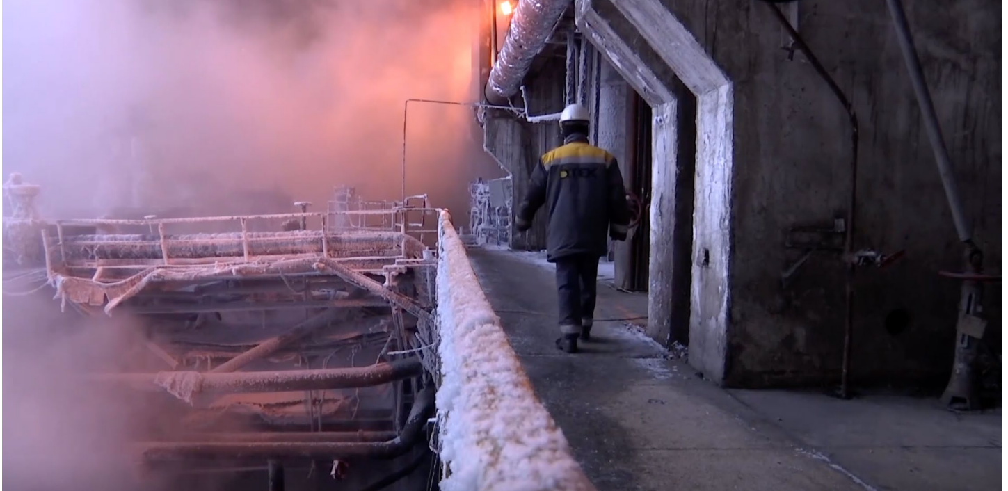
Photo: A centralized heating plant stands frozen after sustaining severe damage from Russian missile strikes. During the overnight attacks on Kyiv on January 21st, Russia targeted the city's energy facilities and electrical distribution centers, leaving large areas without light, power, heat, or running water.
